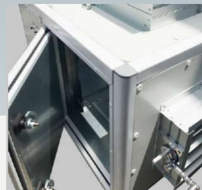
Mixing Chamber Up steam of Filter section.
