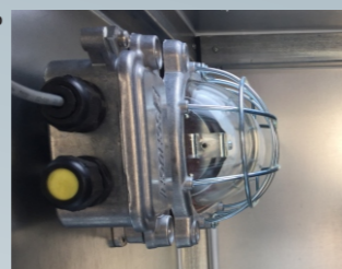
Explosion proof lamp For eliminate risk of explosion, all possible spark equipment shall be minimize risk of explosive.
